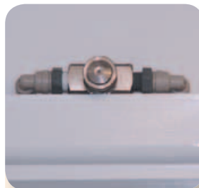
The discreet pipework can be fed through to fit above a door or other non-intrusive area.
